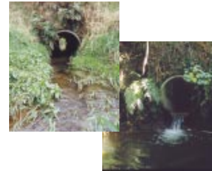
The culvert overhang (at right) will prevent fish passage. The culvert placed at streambed level (left) provides closer to natural conditions all through its length and allows unrestricted access for fish at most flows.
